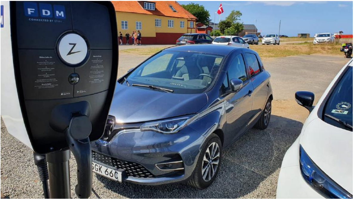
ZAPTEC Pro installed by our partner Spirii in Bornholm, Denmark.
