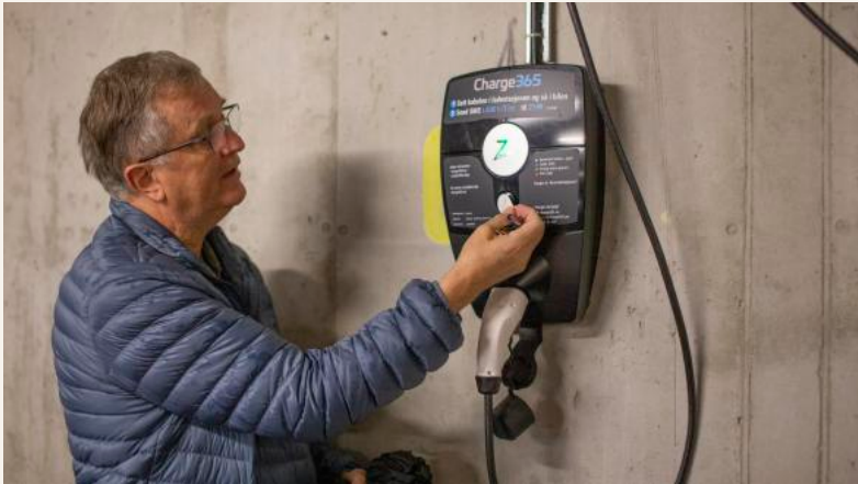
Zaptec Pro charging system integrated with Charge365 payment services.
